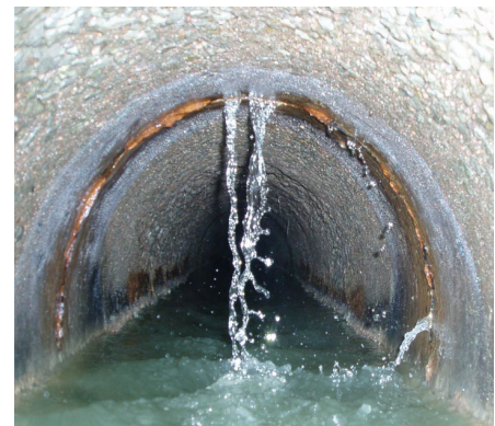
Infiltration Into a Sanitary Sewer
