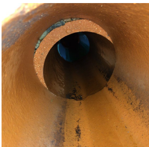
Offset Joint Detected via CCTV Inspection
