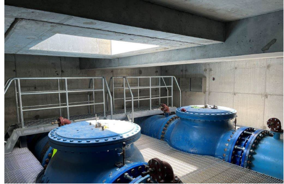
WASM 3 42-inch diameter PRVs
