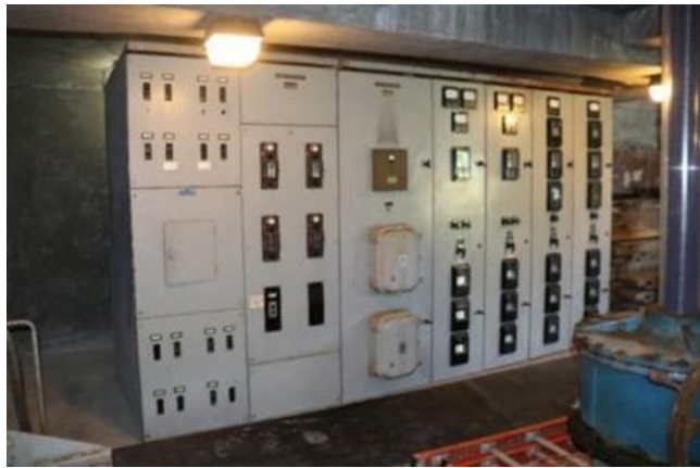
Shaft 5 - Electrical Switchgear to be replaced
