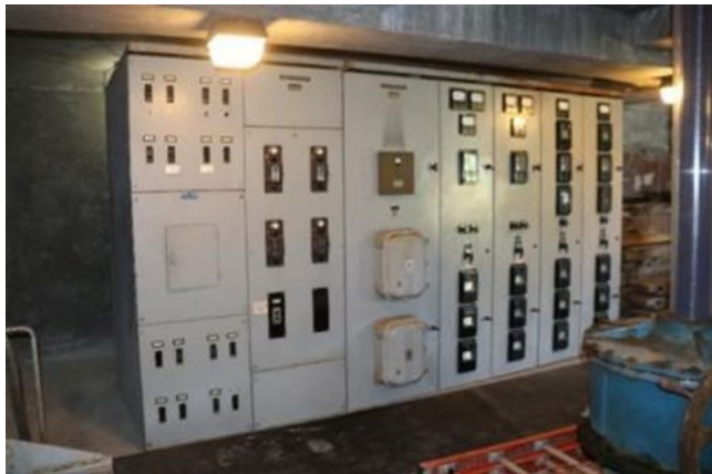
Shaft 5 - Electrical Switchgear to be replaced
