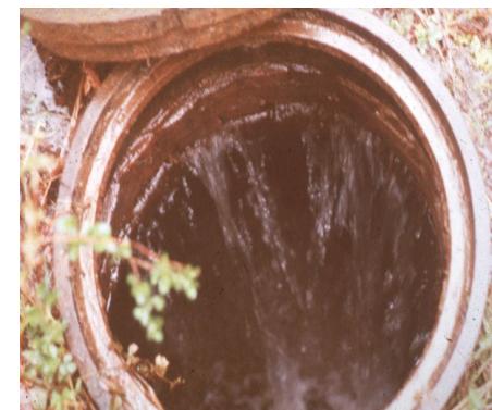
Inflow Into a Manhole During Flooding
