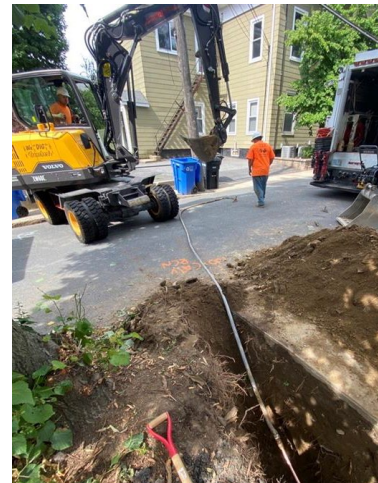
Lead Service Line
