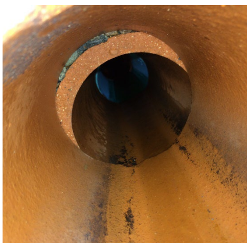
Offset Joint Detected via CCTV Inspection
