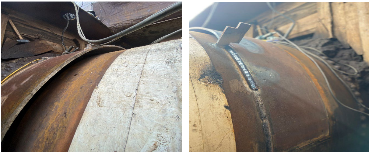
Differences in Diameter at Welding Connections
