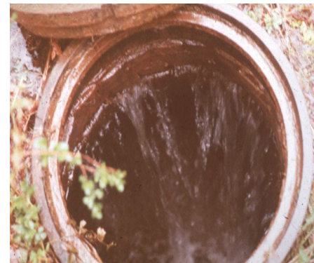
Inflow Into a Manhole During Flooding
