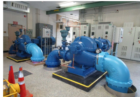
New Pumps at Commonwealth Avenue
